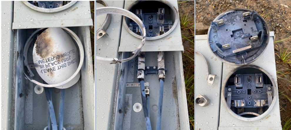
Factory provided meter ring left inside meterbase
