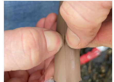
In this picture the blade cut deep into the insulation, which then required the contractor to re-terminate. An improperly adjusted tool can cause a lot of wire damage, which could require contractor to re-pull wire.
