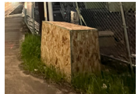
Recent example: contractor installed a plywood box over 1/0 ug primary to avoid theft/ damage in a high traffic area.
