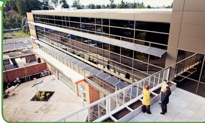
HeLa High School solar array - innovative installation generates renewable energy and provides shade
